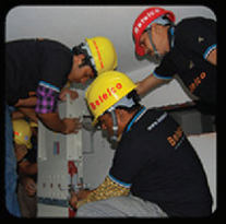
BBT installation at BRB Hospitals Limited Panthapath, Dhaka, BANGLADESH
